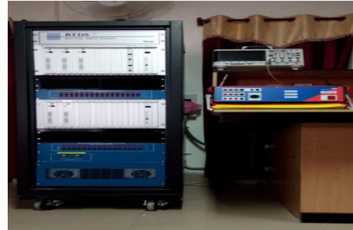
ADVANCED POWER LAB
