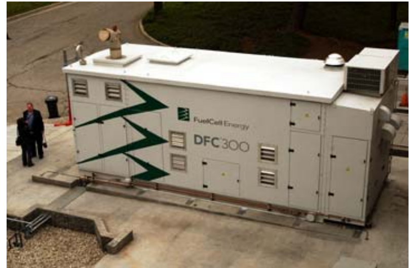
While barely the size of a tractor-trailer, Los Angeles' John Ferraro Building Fuel Cell Power Plant provides enough energy for 250 homes.
