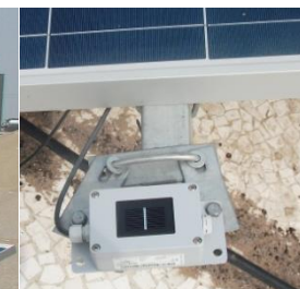
Pyranometer and Irradiance sensors with module temperature sensor
