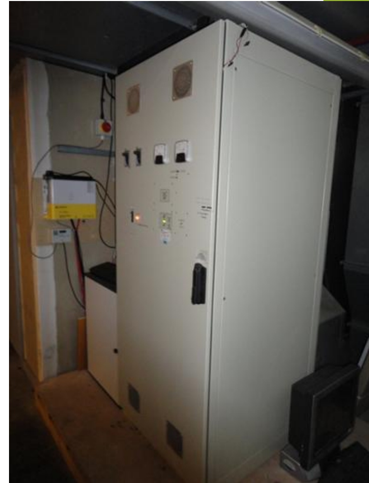
AC-DC converter and battery management controller
