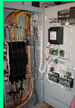
Switchgear, Relays, & Controls
